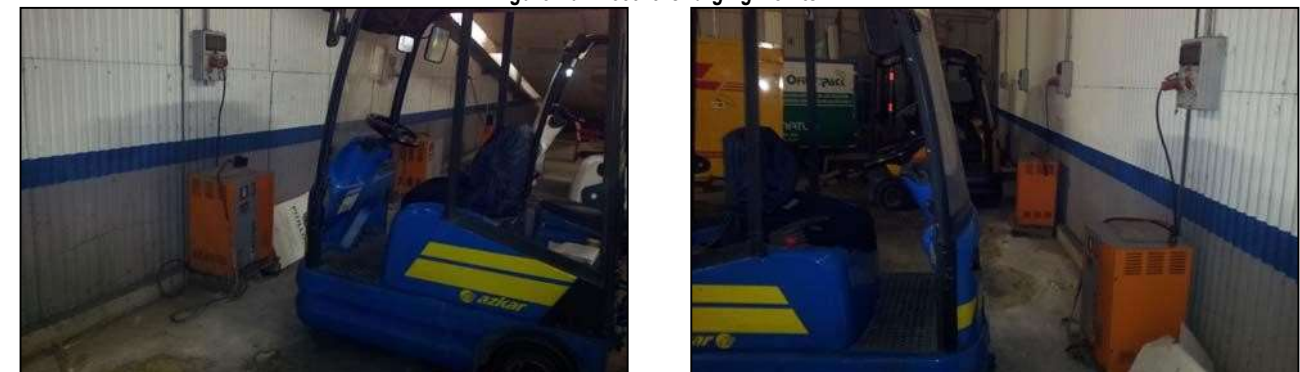
Figure 20. Electric Charging Points.
